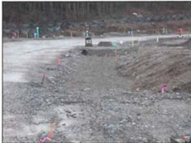
Figure 8: The rock trench, perforated drain and overflow should be constructed at the same time as other subdivision utilities.
