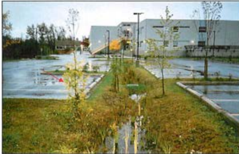
Figure 4: The overflow drain height should be set to allow for temporary ponding during high intensity events.
