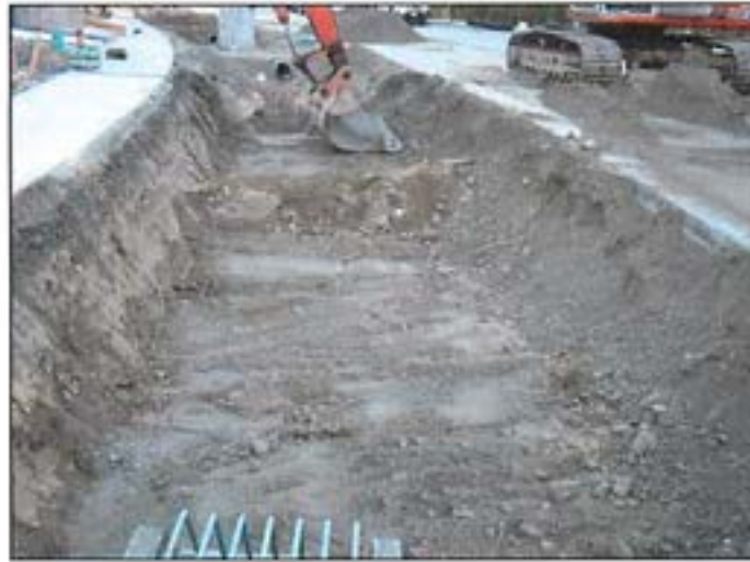
Figure 12: The sand layer may need to be scarified before adding the growing medium to the rain garden.
