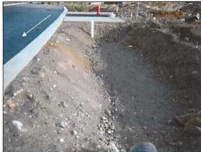
Figure 14: Minor flows can be contained along the panel curb prior to the second lift of asphalt.
