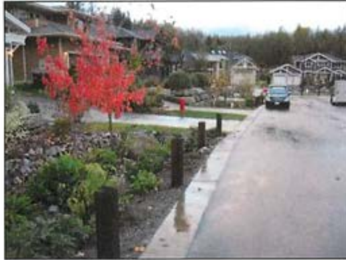
Figure 10: Growing medium and plantings should be put in after buildings are complete (but before the second lift of asphalt).
