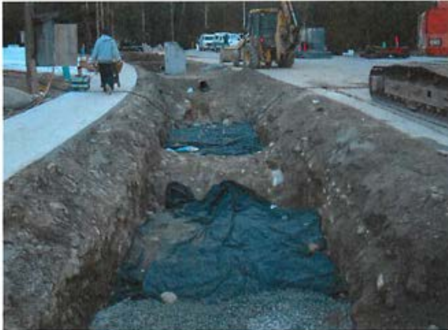
Figure 7: When communities are built, utility trenches are constructed and perforate the site. If the rain garden trench extends too far below the invert of the major utility trenches, the theory is that infiltration rates will tend to decrease.
