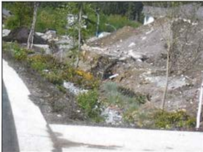
Figure 11: Growing medium and plantings should not be put in before building construction is complete because stockpiled material may get into the garden and smother the plants.
