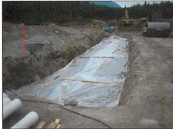
Figure 9: The rock trench should be protected with a sacrificial soil layer and poly sheeting while roads, driveways, sidewalks, and buildings are constructed. Once covered, the depression can be used as a settling facility for lot runoff then removed once the lot is completed. 2 x 4s can be used on top of the poly to assist in the location of the poly upon removal of the sacrificial material.
