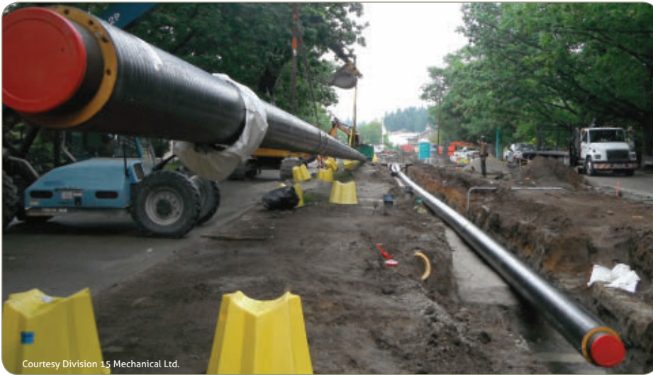
Installation of 16-inch preinsulated hot water distribution piping, University of British Columbia
